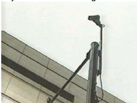
(a) The camera unit is typically mounted at a height of 9m to maximise the "field of view".
