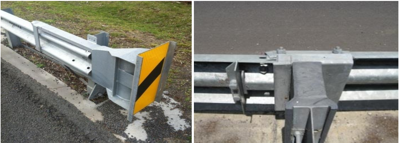
Figure 2. Incorrect installations from Cassar (2015)
