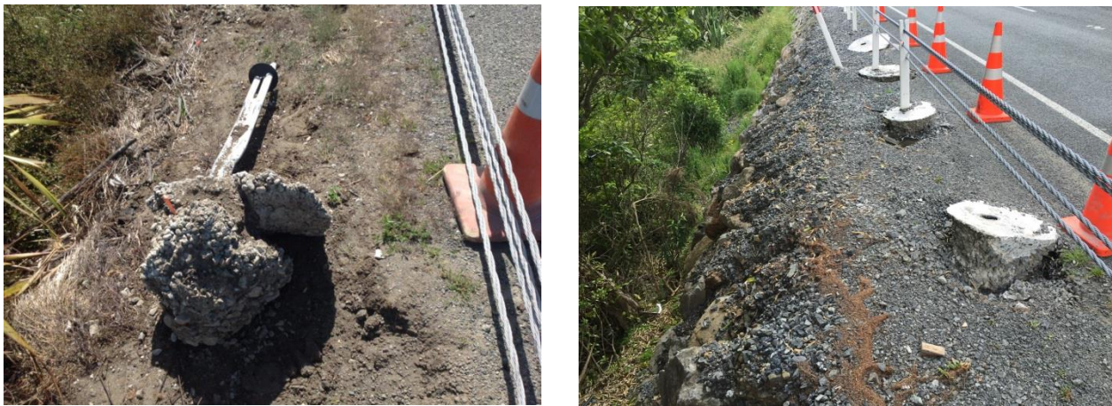
Figure 1. Post failures shown in NZTA TAN 16-01
