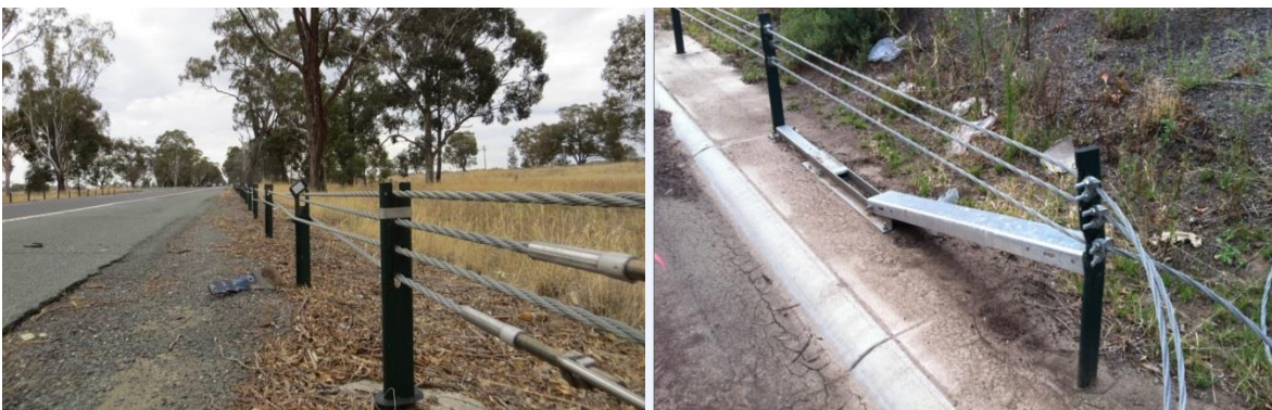
Figure 4. Inappropriate wire rope barrier installations from Cassar (2015)
