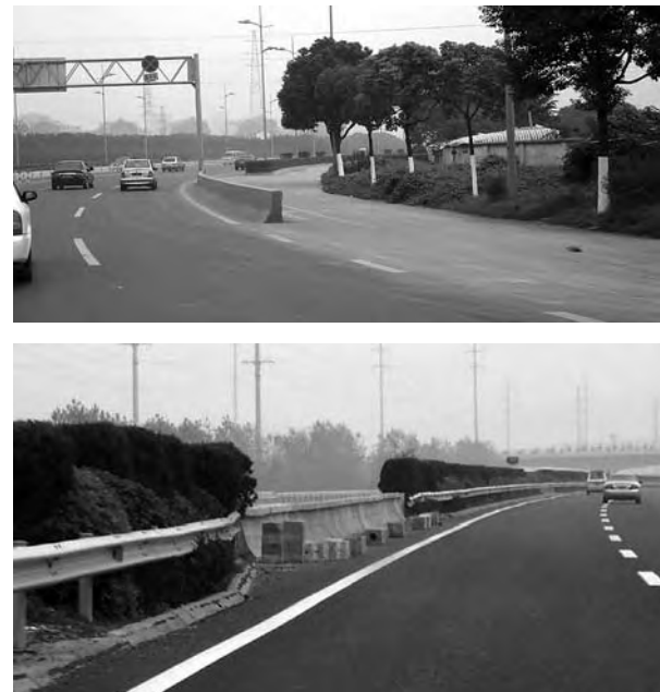
Figure 4 - Top: 80 km/hr zone with blunt end barrier with no crashworthy end terminal. Bottom: block of concrete placed in front of W-beam guard rail ends with no terminals on 100 km/hr tollway.
