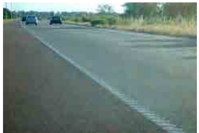
Tactile strips on line markings can provide audio warning to motorists
