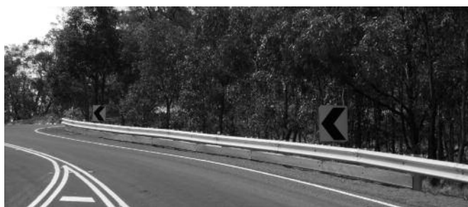
Below: Rub rail to prevent motorcyclists crashing under the barrier
