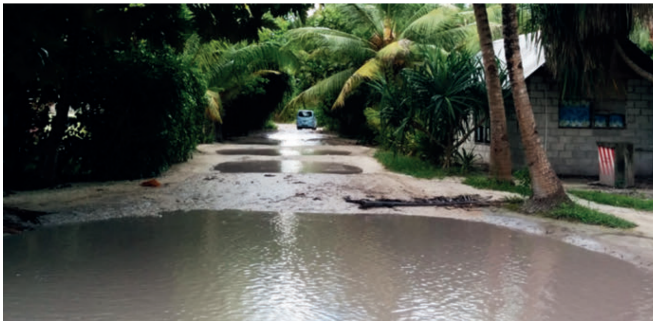
Figure 2. Poor condition of South Tarawa Road prior to the KRRP
